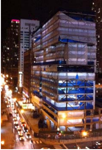
Oxford Capital is developing The Godfrey Hotel, which originally was designed as a Staybridge Suites before the project's first developers defaulted midway through construction.
